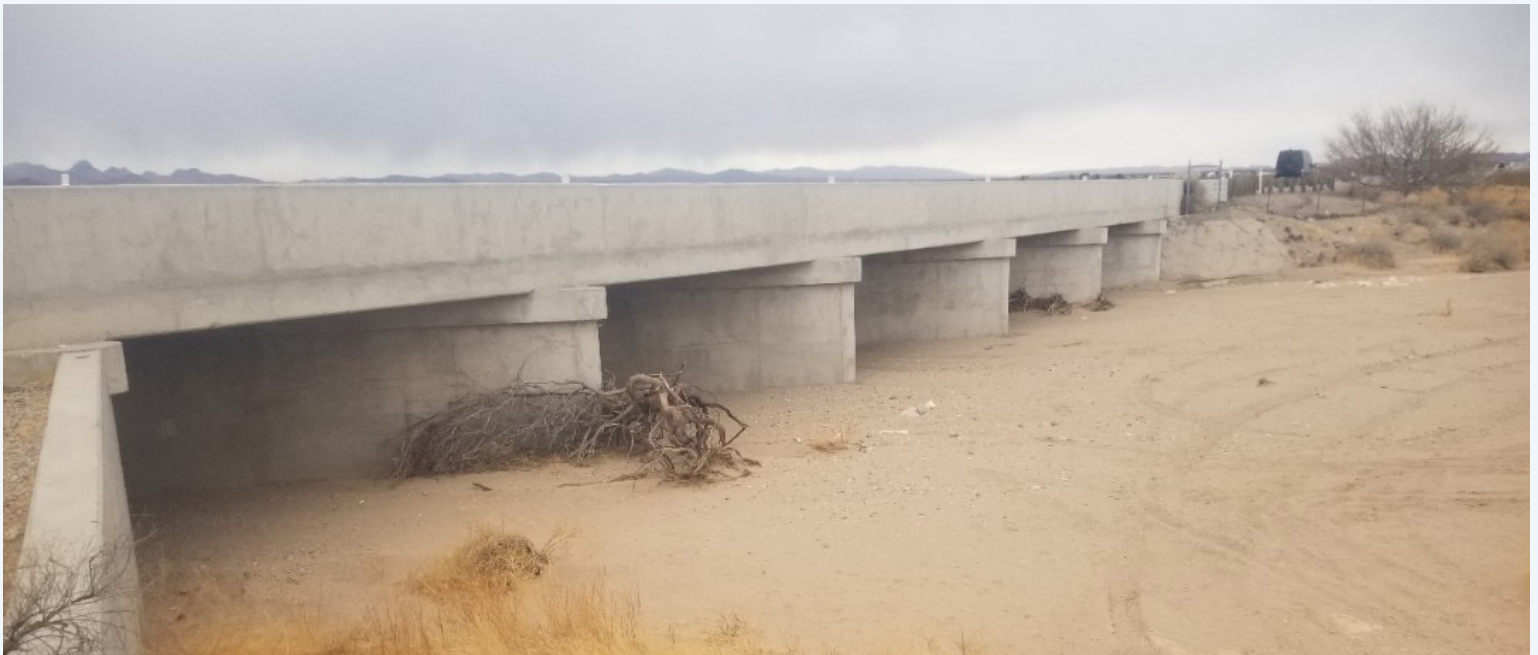
An example of a highly accessible culvert for desert tortoise use.
